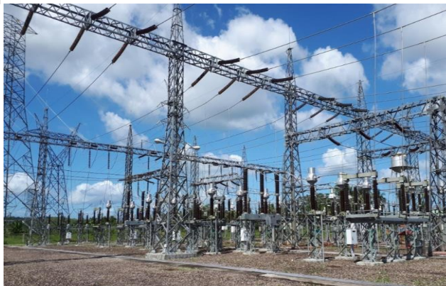
NGCP (Philippines Electricity Generator)
